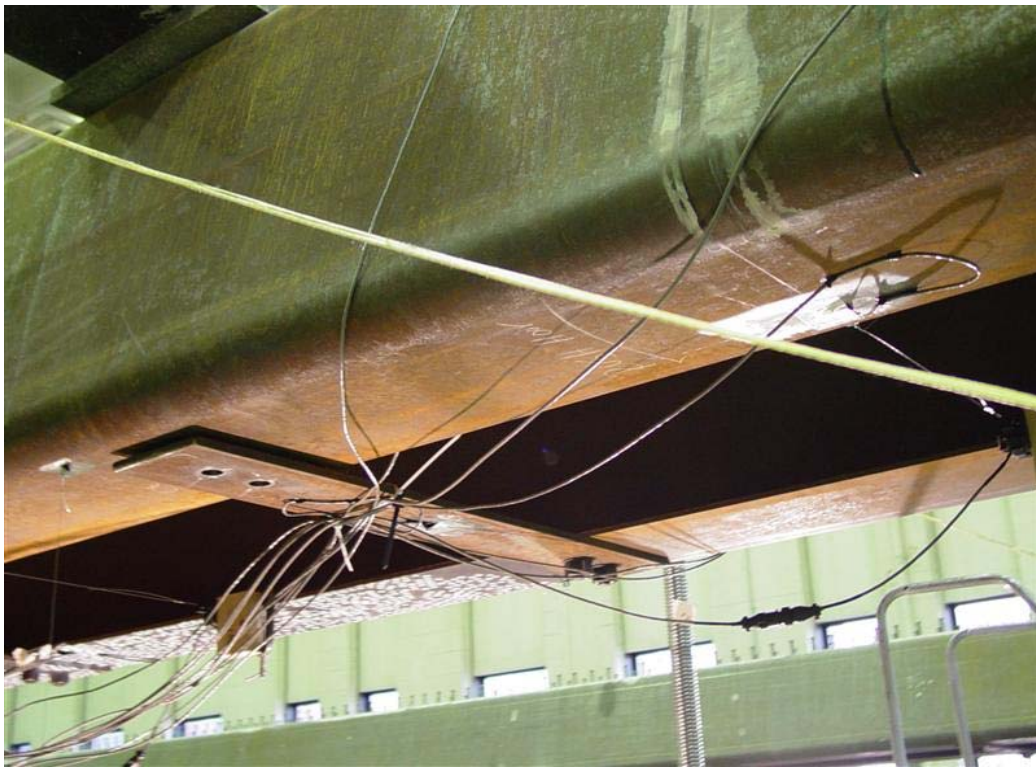
Figure 2-13 Disconnected tie plate at section H
