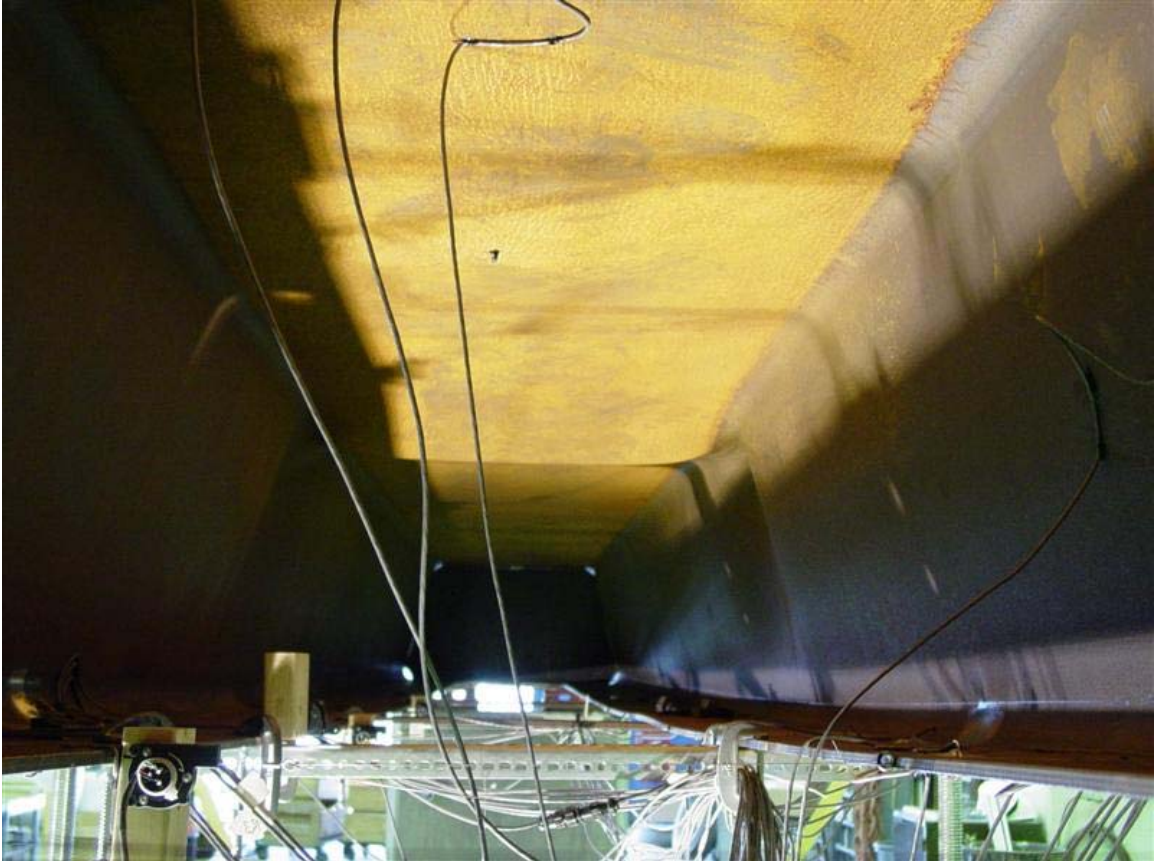
Figure 3-10 Inside of folded plate girder after failure
